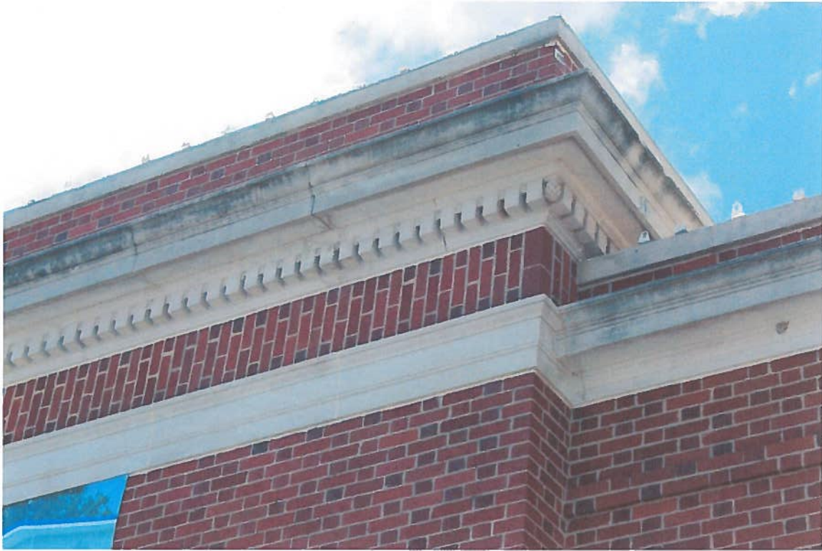
View south façade at change in roof elevation. Detailed cast stone cornice on left is over lobby area. Lower roof is over mail sorting floor (gallery space).
